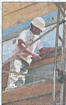
Jeff Rivenbark, owner of Rivenbark Masonry, lays a course of bricks at the Culpepper Construction project.
